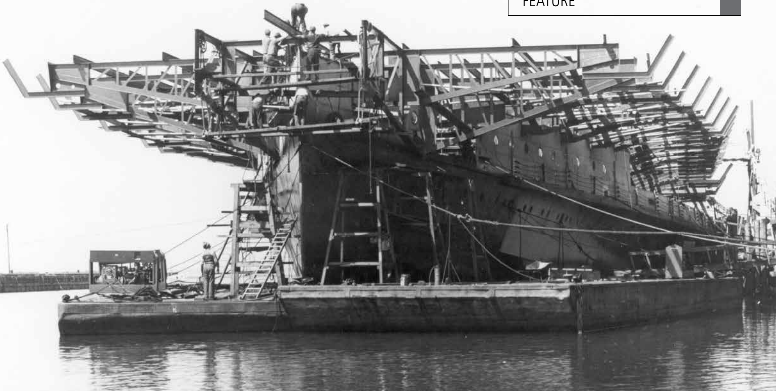
The USS WOLVERINE (IX-64) being converted from SS Seeandbee at Buffalo, New York, on June 12, 1942. A wood plank deck would be installed over the steel structure that was refitted atop the luxury paddle-wheel steamer. Official U.S. Navy photograph, now in the collections of the National Archives.
